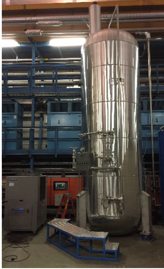
Figure 4: Recovery and Storage system of Xenon (ReStoX2) for XENONnt after installation, in July 2018, at LNGS.
