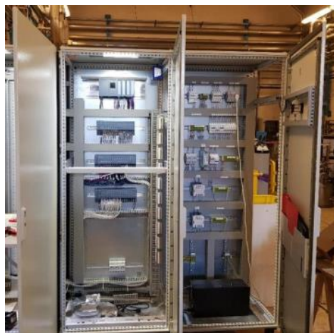
Figure 11 : Picture of the cabinet assembly at IJCLab dedicated to cryogenic controls and interlocks.
