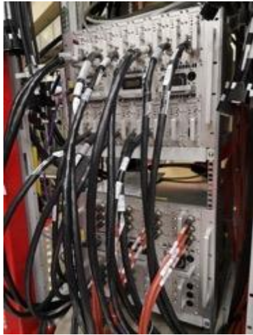
New LVPS group for 8 ATCS New LVPS installed on Profibus.
